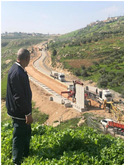
Watching a new sector of the Separation Wall being built in Sheikh Sa'ed
